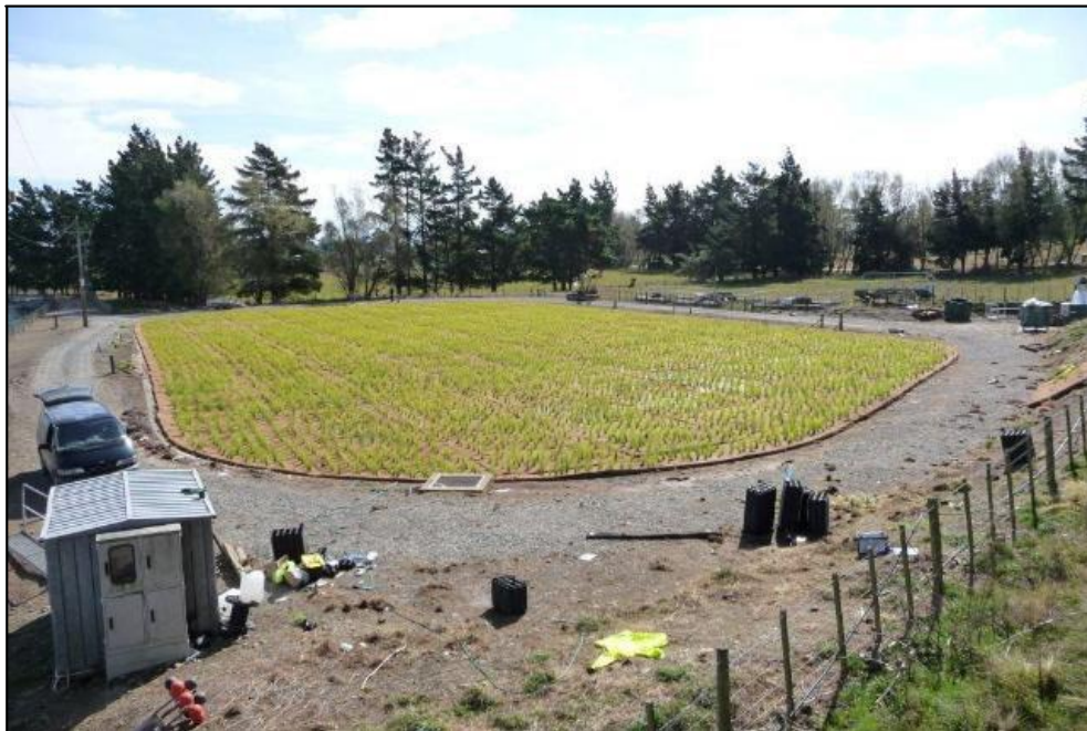
BioHaven serving as wastewater lagoon blanket
